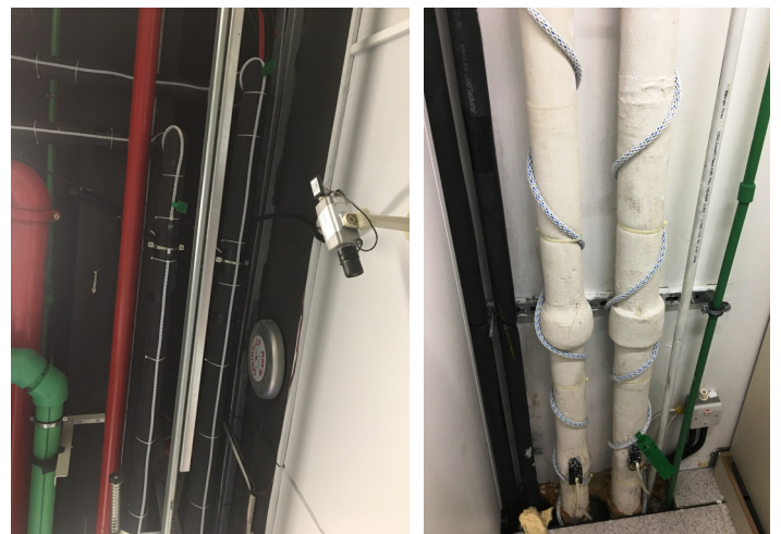
Horizontal & vertical chilled water pipes equipped with FG-ECB cables
