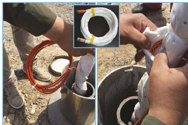
Figure 3. An example of an installation with monitoring wells, able to cope with pre-existing soil pollution.
