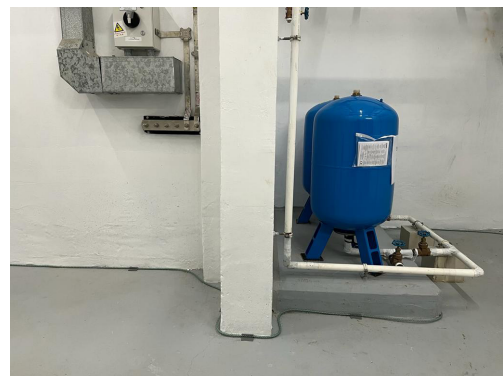
TTK addressable sensing cable installed close to a pump
