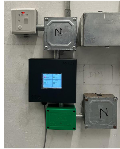
FG-ALS4 local monitoring panel and FG-DTM Modbus Interface installed on site
