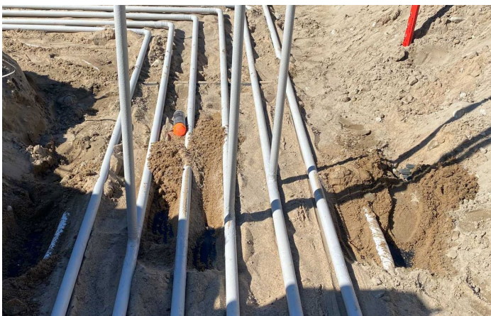
On-site fuel pipelines
