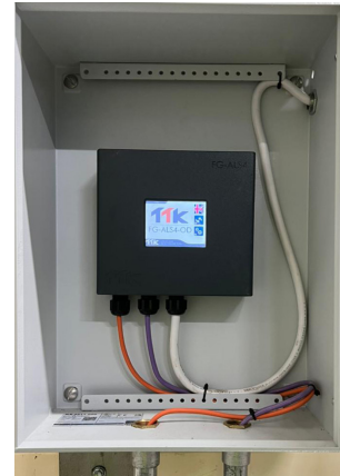
Four Zones Alarm & Locating System Unit for Hydrocarbon Leak Detection (FG-ALS4-OD) installed on site
