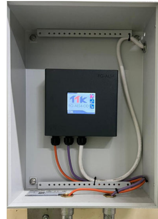
Four Zones Alarm & Locating System Unit for Hydrocarbon Leak Detection (FG-ALS4-OD) installed on site
