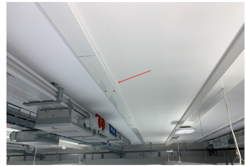
Ceiling ducts and TTK sensing cables run inside
