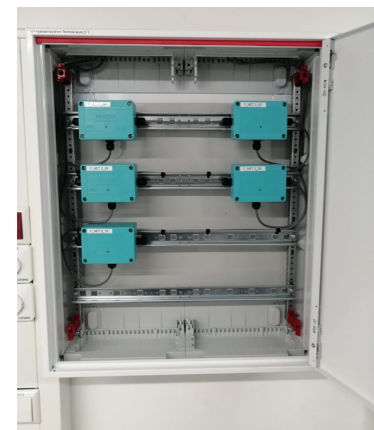
TTK diversion boxes (FG-DTCS) inside a specific enclosure
