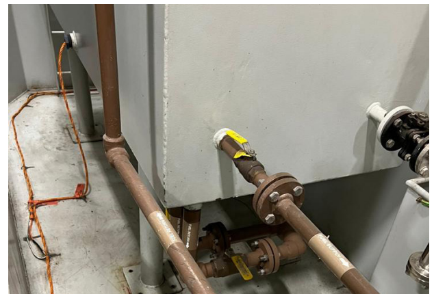
TTK Hydrocarbon Sensing Cables Installed Near Fuel Pipes
