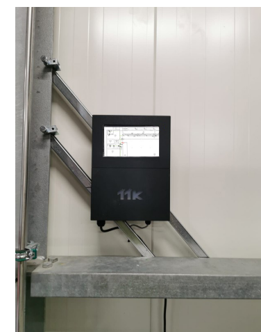
FG-NET digital monitoring control panel installed on site
