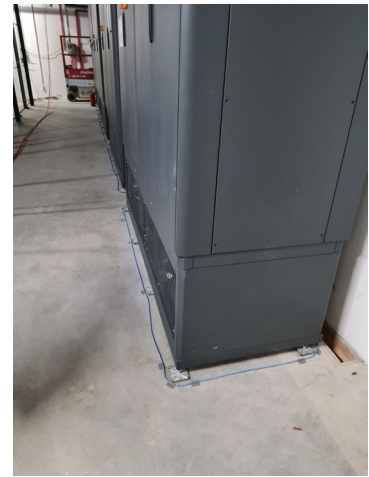
FG-EC Addressable water leak detection cable installed around CRAH unit
