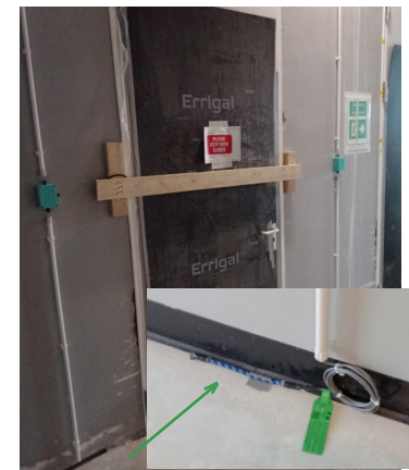
TTK customized L-shape water point sensor (FG-ECP) near a corridor door
