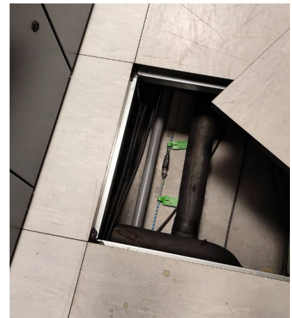
TTK water sense cable installed under the raised floor, alongside the pipework
